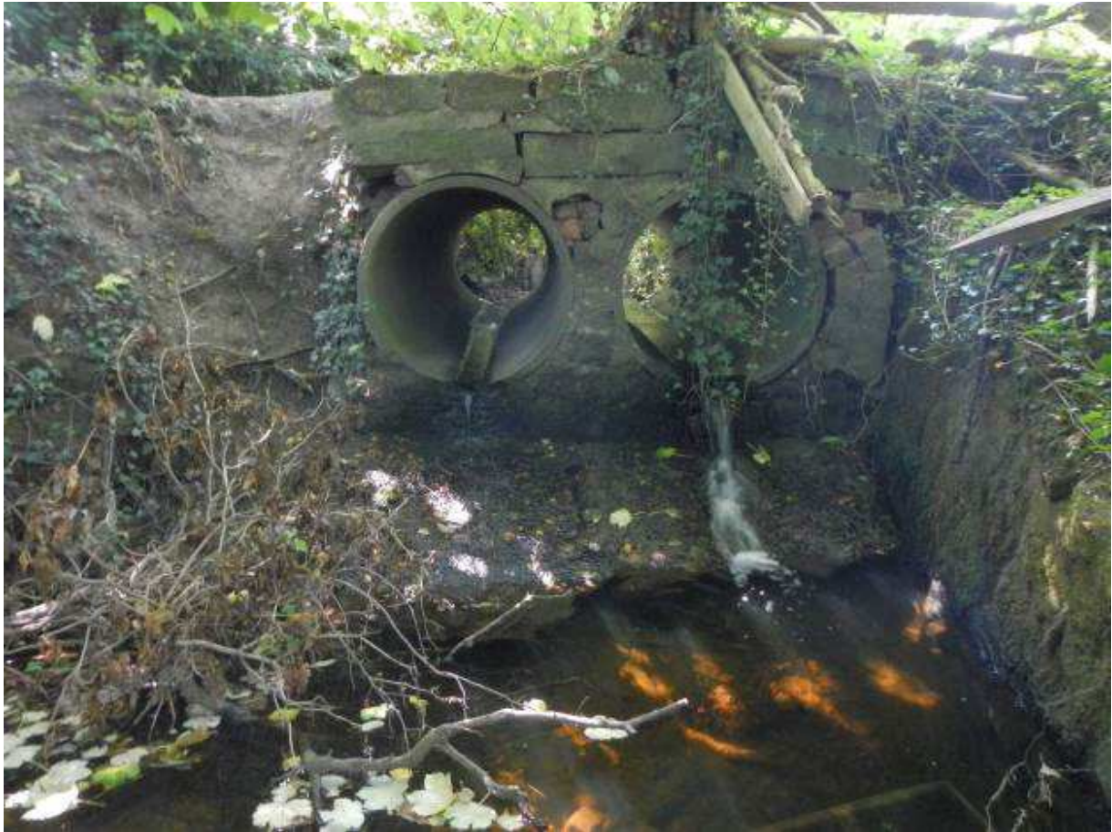
Figure 4. Perched culvert making access to the Backstone beck impossible until rising river levels increase the tail-water level and begin to decrease the height differential. This does not necessarily mean that main river trout will not run the beck, when conditions allow, or remove the potential for resident beck fish contributing to the River Wharfe population.
