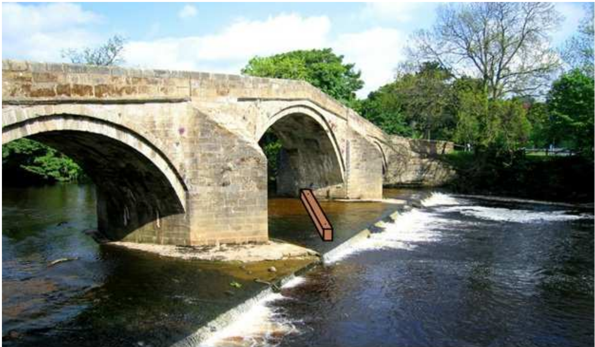
Figure 8. A simple diagonal baulk located in the centre bridge arch would increase water depth and aid fish passage.
